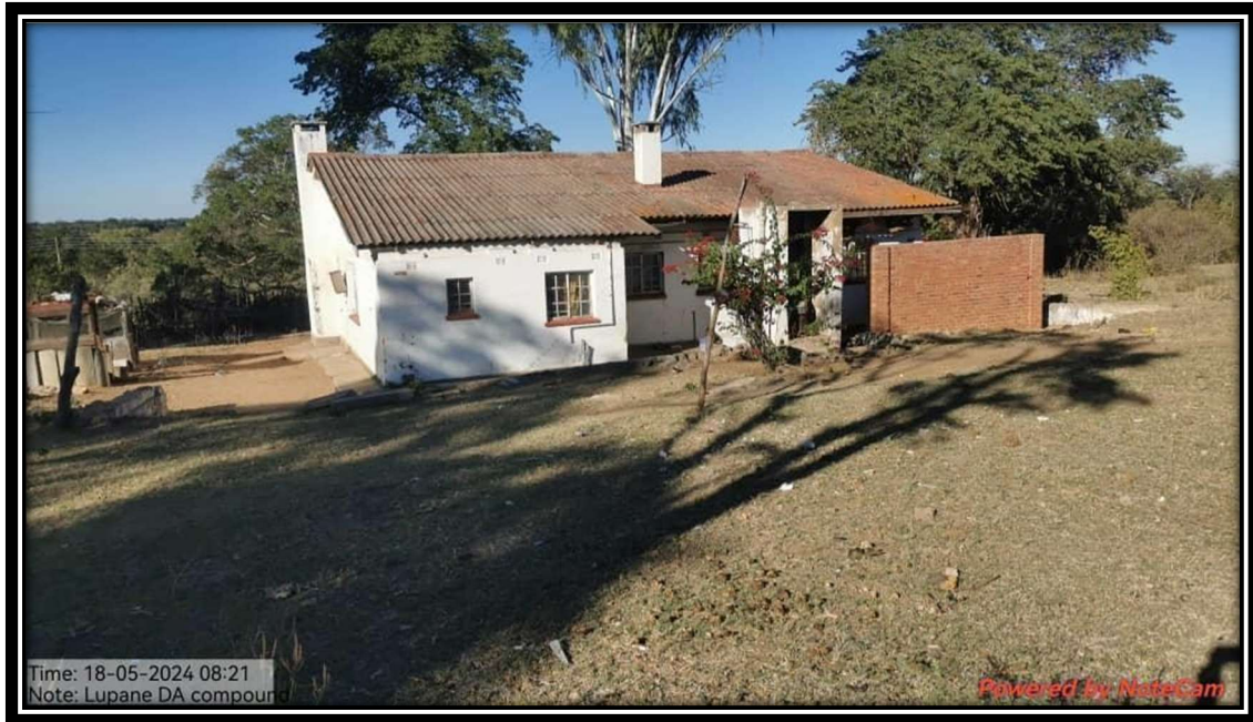
Plate 6.1: Dilapidated Housing Units at the DA Compound
